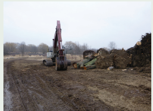
The project will incorporate salvaged large woody debris for bank stabilization and habitat structure
