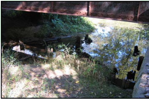
Sediment Deposited Below a Railroad Bridge
